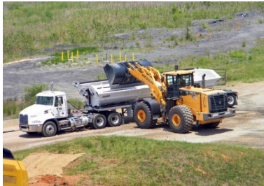
Coal ash stored at Duke's Riverbend power plant is loaded for transportation to a landfill. Source: Duke Energy
